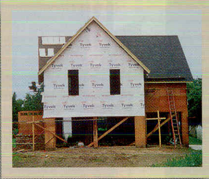
The carriage house was built to replicate the original structure, as documented in photos. Today it serves as a garage, providing both form and function for the Ruppman's.
