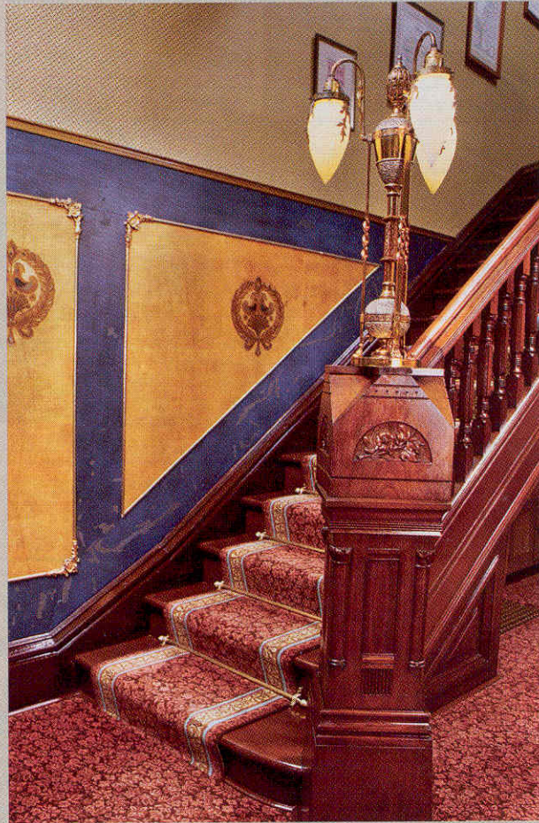
Reconstructing this staircase was a major project. Though narrow and steep, restoring it helped the house regain its original character.
